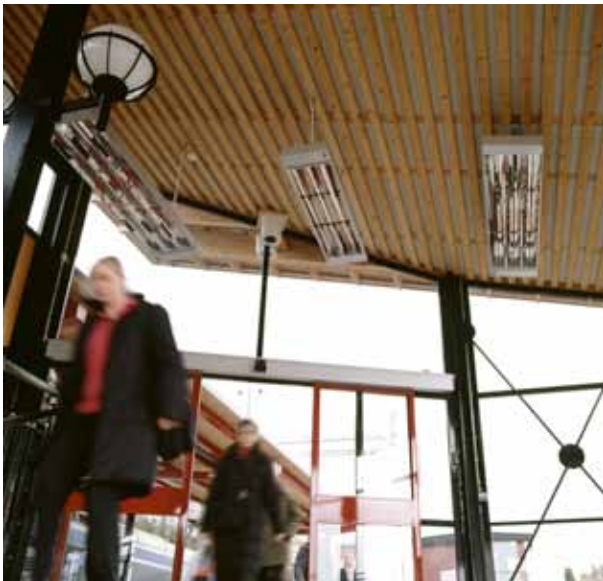
This train station outside Stockholm is heated by IR. A control with timer allow waiting passengers to increase the heat when it is particularly cold.
